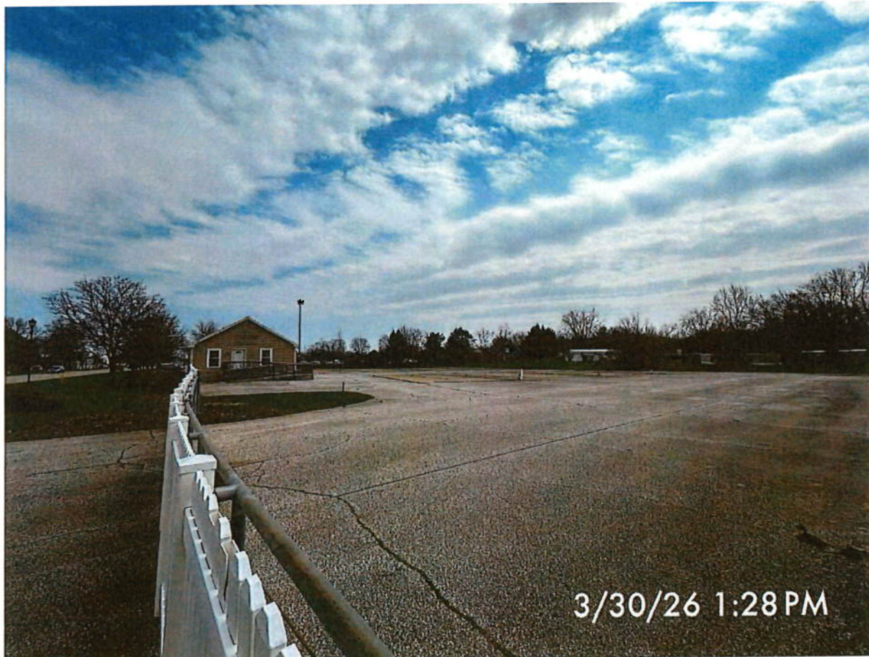
P5. Looking westerly from the access drive toward existing paved area south of building.
