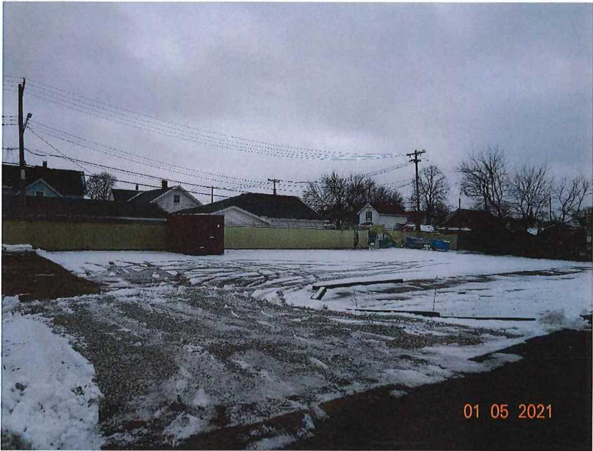
Rear parking lot of 411 S Main. Gravel to be removed or made hard surface.
